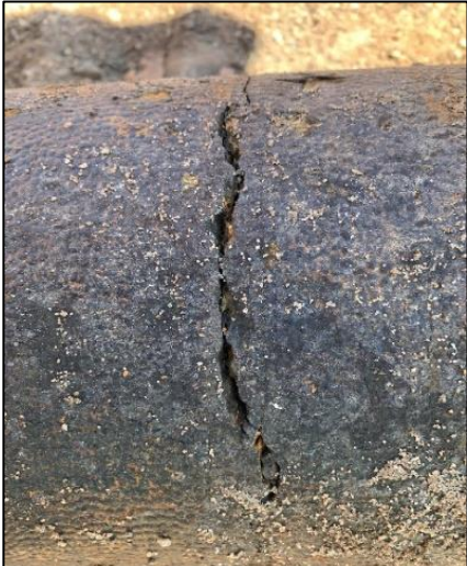
The crack found in watermain that resulted in emergency water shut-off
