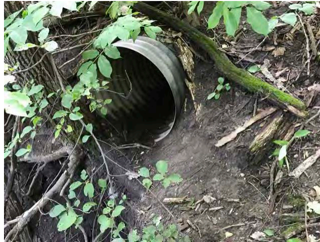
Photo 15: Culvert that feeds Erosional Feature 2
