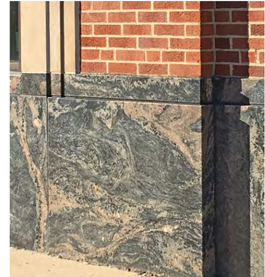
Stone and brick, as on the Marshalltown Police Building, is an example of authentic materials.
