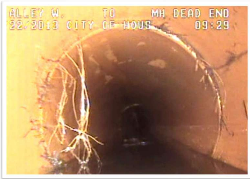
Exhibit 4 – Root Intrusion Through Pipe Joint. West of Washington Street
