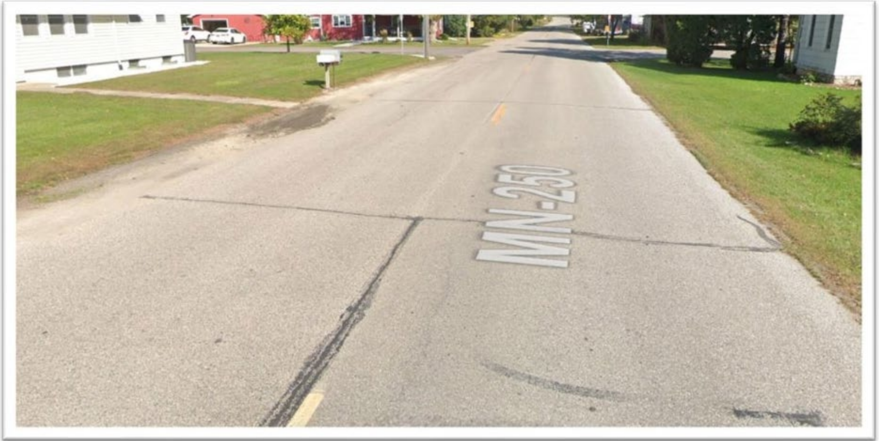
Exhibit 3 – Ashburn St E Road Conditions
