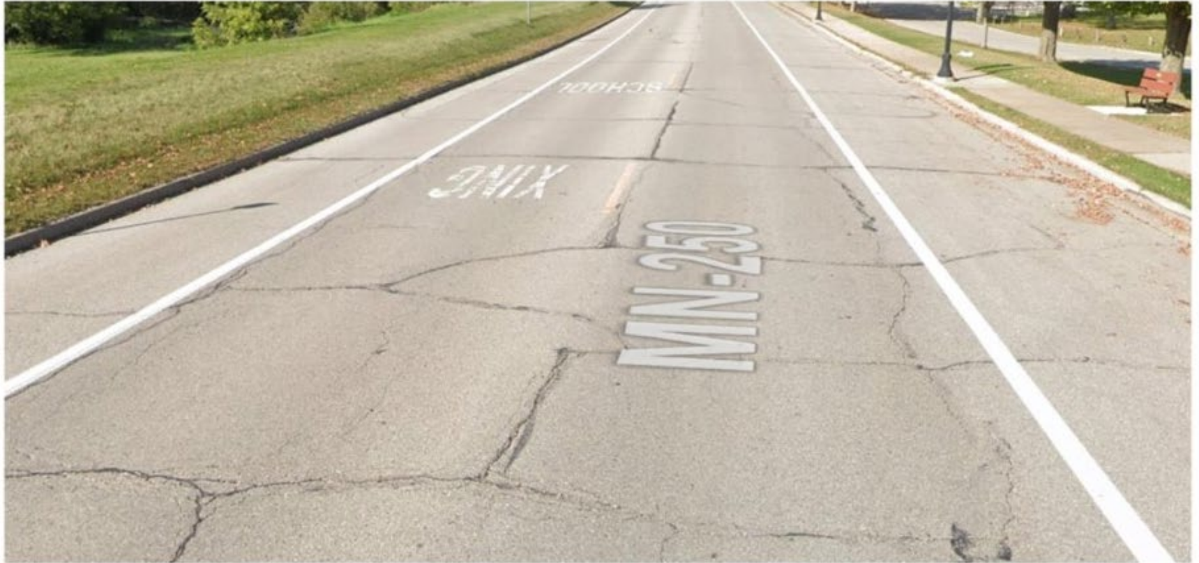
Exhibit 1 – Parkway Avenue South Street Condition
