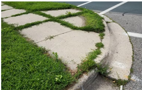
A non-compliant pedestrian ramp with vertical discontinuities greater than 1/2 inch, vegetation growing through cracks, and no detectable warning such as truncated domes.
