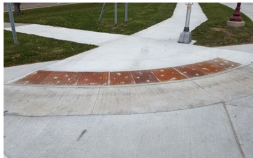
An ADA-compliant, blended transition or fan, pedestrian ramp with truncated domes and easy access to the pedestrian access route.
