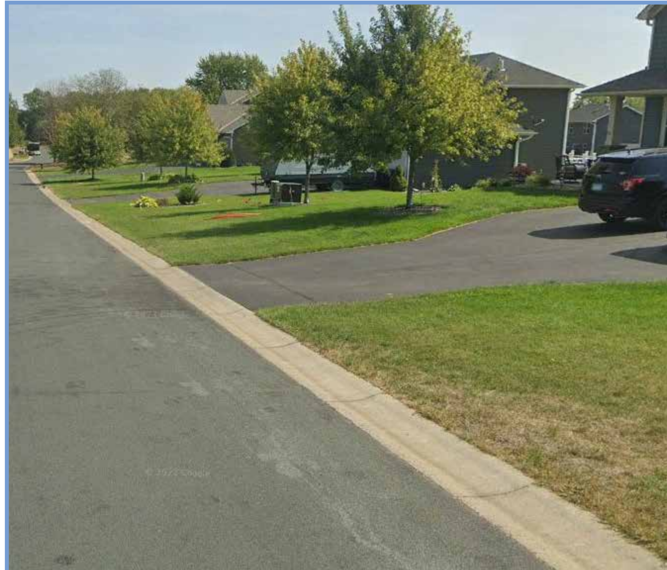
SURMOUNTABLE STYLE CONCRETE CURB
