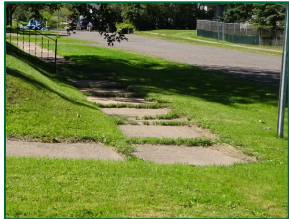
Proctor sidewalks in a state of broken disrepair.
