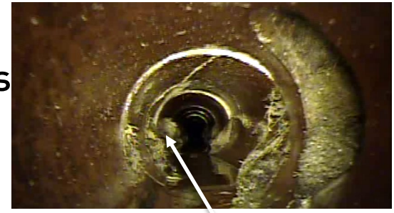
Roots Growing Through Pipe Joints
